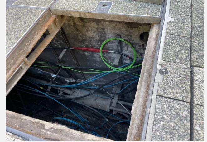
Protection of communication pits
